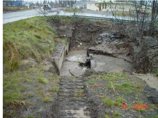
Homer Storm Flood Damage
